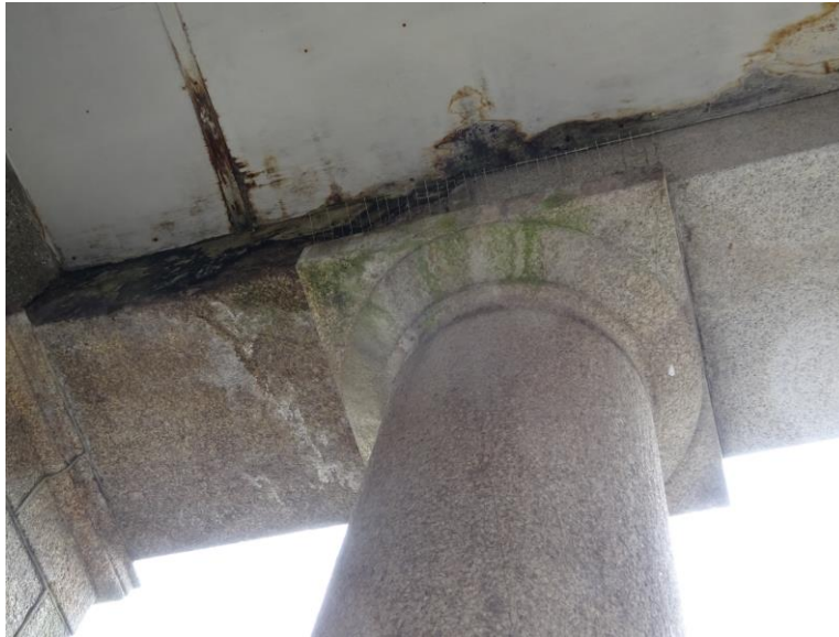
25. Delaminating lintel over column.
