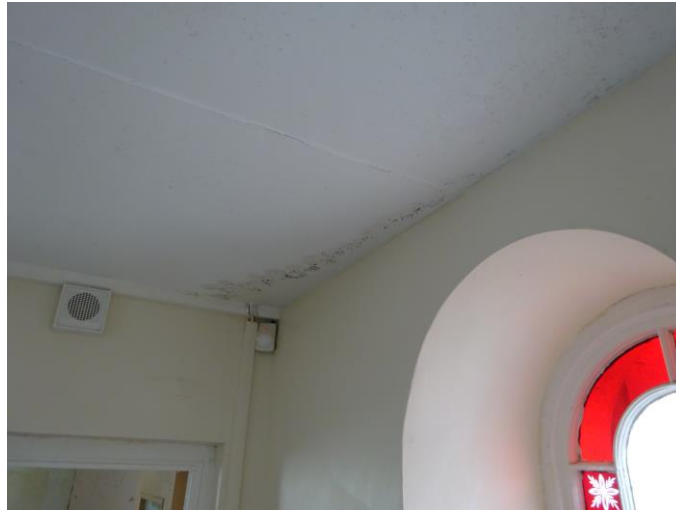
42. Damp stain to east corridor north side.
