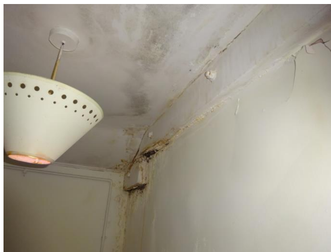
46. Damage to ceiling / wall accessible lavatory north side.
