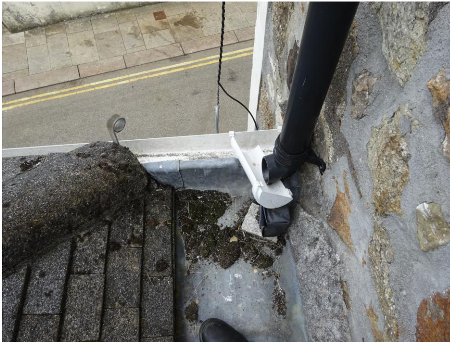
21. Poor downpipe outlet detail to northwest corner of western hall.
