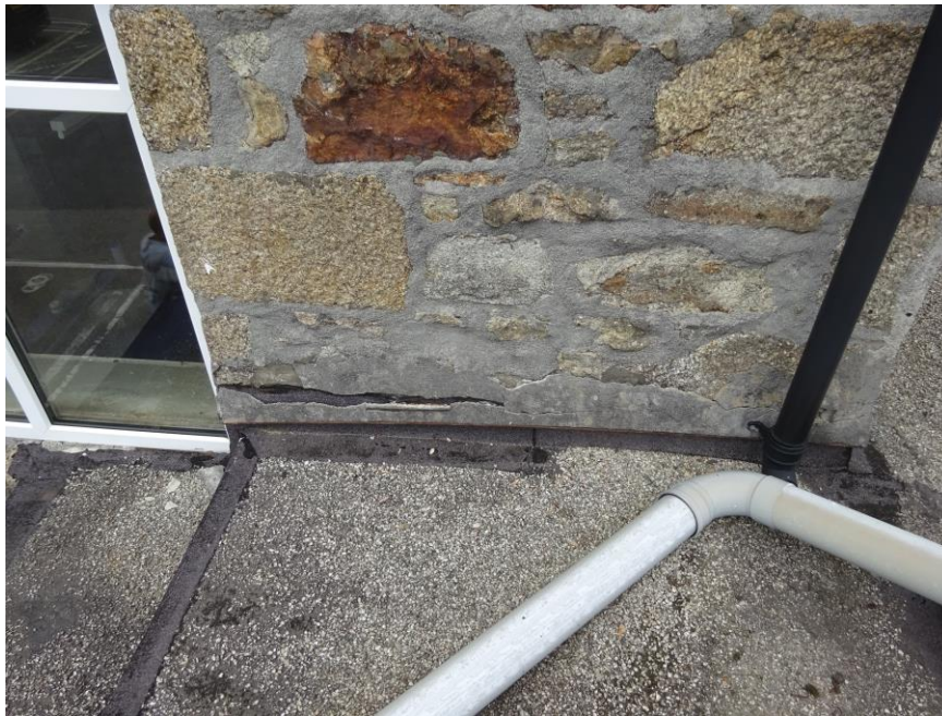
28. Defective weathering from flat roof to Wall 8.
