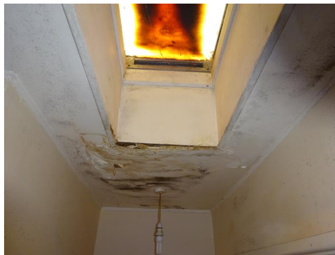
13. Internal water ingress from flat roof skylights.
