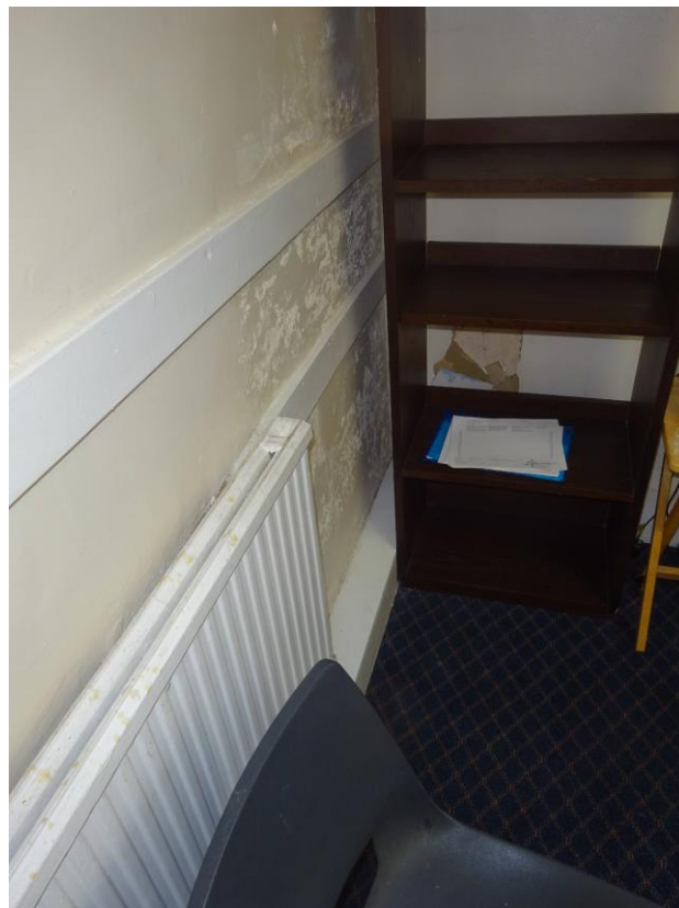
44. Dampness to infill hall due to defects at downpipe.
