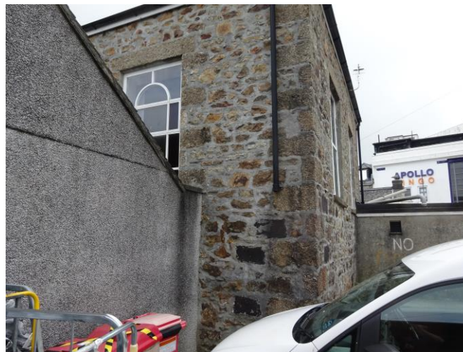
18. Missing downpipe sections southwest corner.
